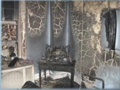
Room at Park Haven Nursing Home where a fire on March 4, 2012 caused by a meth lab in the room killed one person and injured six others
